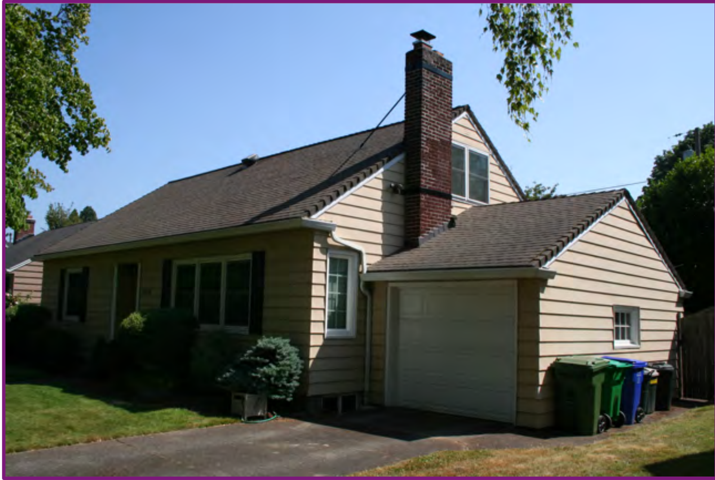
1942 North Portland House Wood frame NOT attached to foundation.
